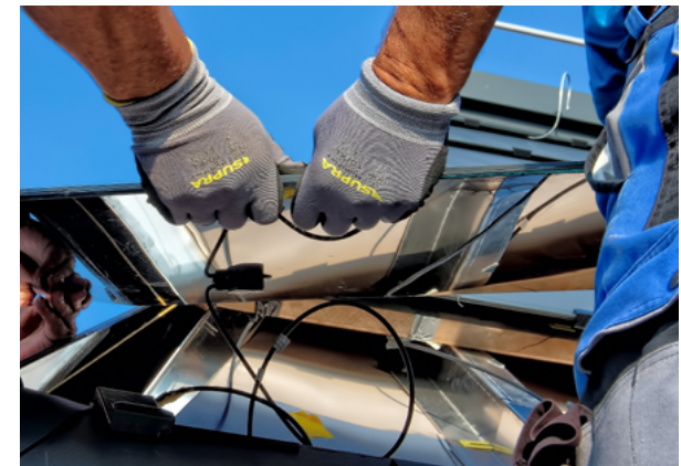
↑ Photo of PV installation by © Ricardo Gomez on Unsplash
